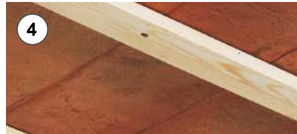
4 - Fissaggio listelli con viti e tasselli 4 - Wooden lath fixing by screws and dowels.
